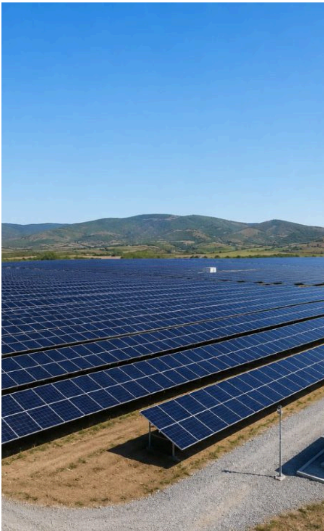
PV SOLAR PARK 49 MWP · SHTIP, NORTH MACEDONIA
